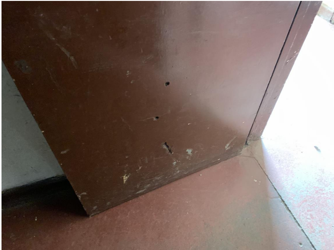
Photograph showing typical example of a door to base to one of the changing rooms.
