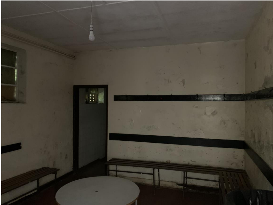
Photograph showing extensive contamination of plaster and de-bonding of paint coatings. Also extensive staining and discolouration noted to walls.
