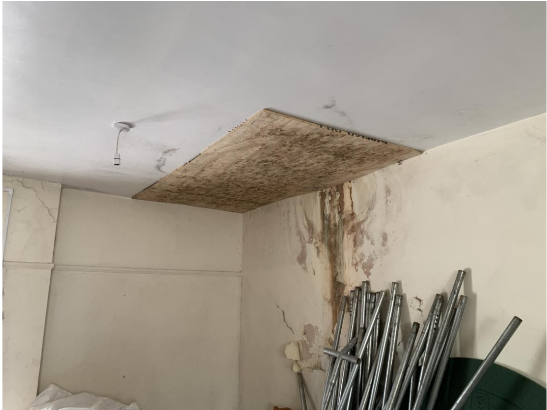
Photograph showing example of water damage to ceiling to the front reception/bar room area.
