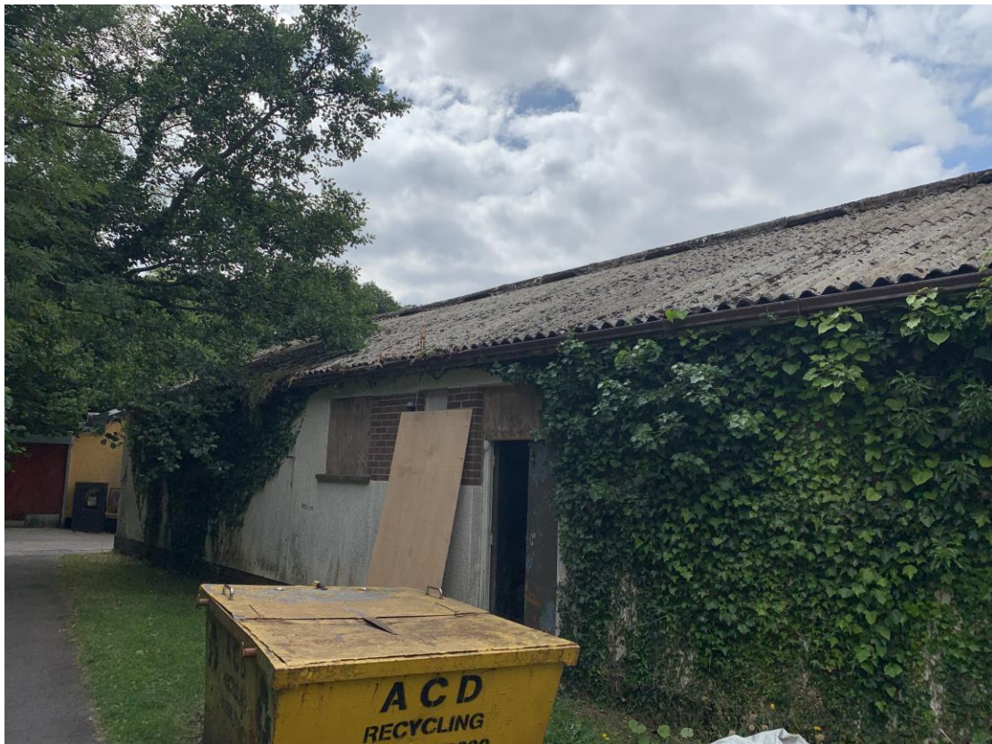
Photograph showing part view of rear elevation where UPVC guttering was noted subject to extensive debris and vegetation growth.
