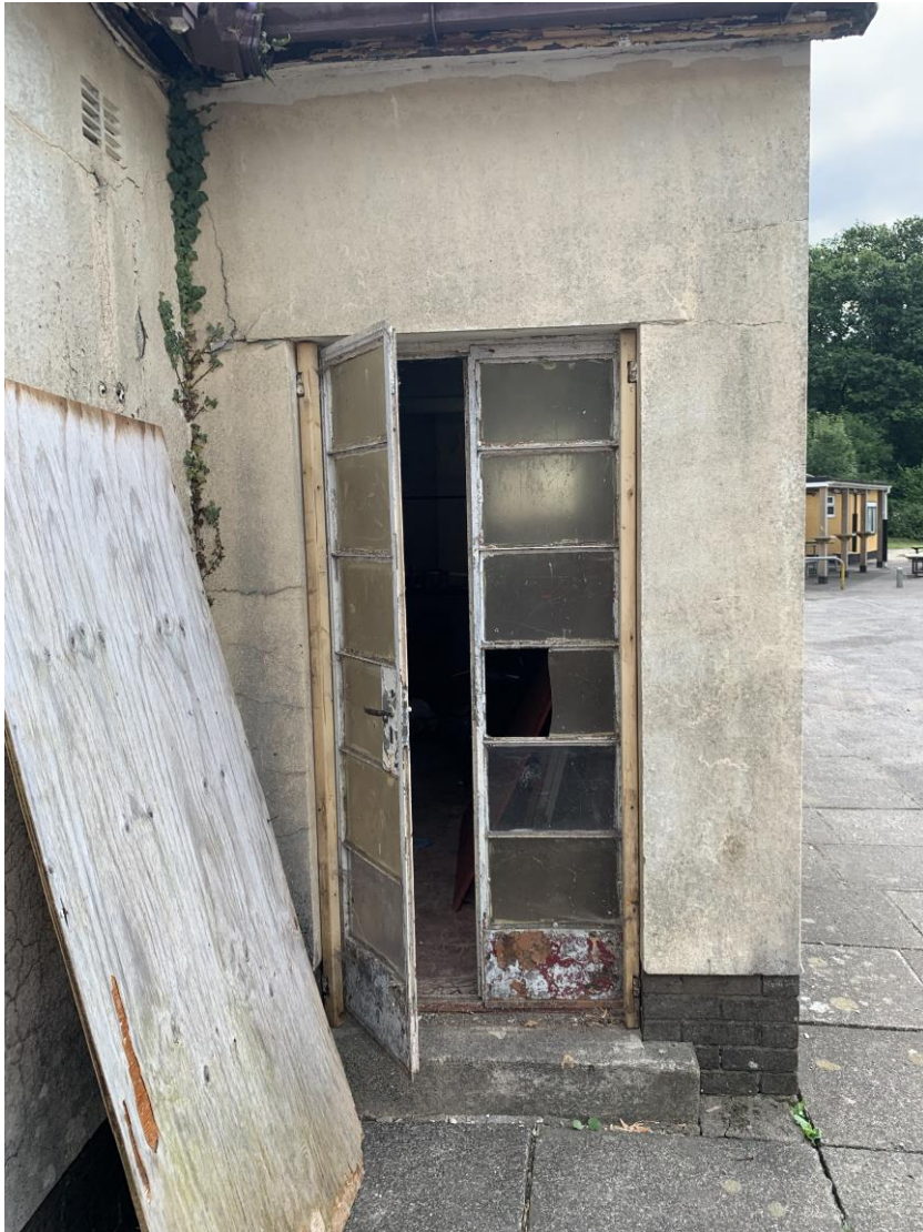
Photograph showing example of the poor condition of the steel crittall single glazed doors to front reception room.
