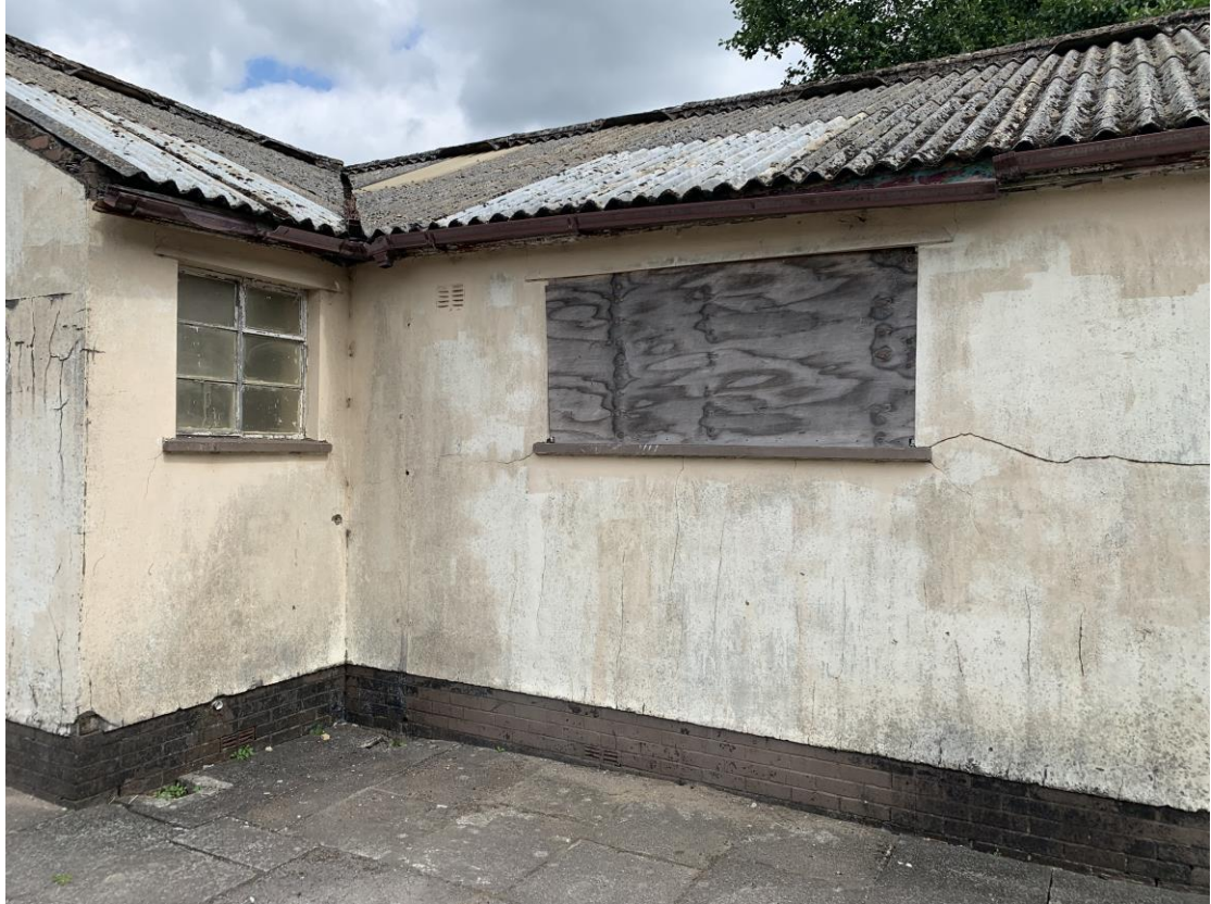
Photograph showing part view of the right side of roof to front. Previous patch repairs and impact damage noted.
