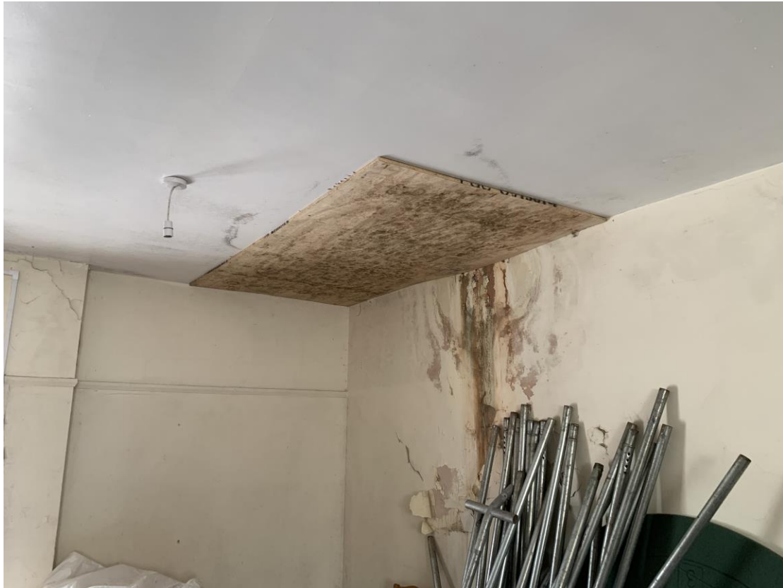
Photograph showing one area where water ingress was noted to the front reception room.
