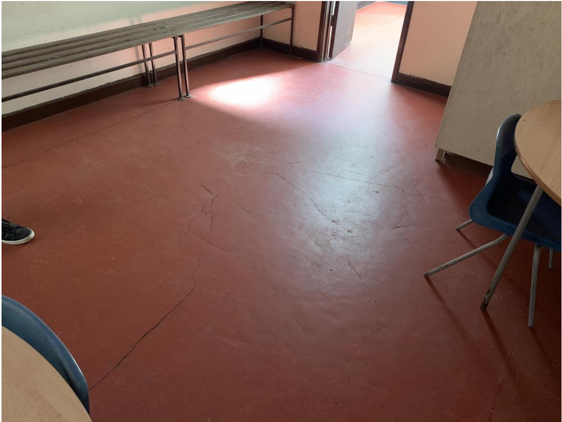
Photograph showing example of undulations and cracking to the flooring to changing room area.
