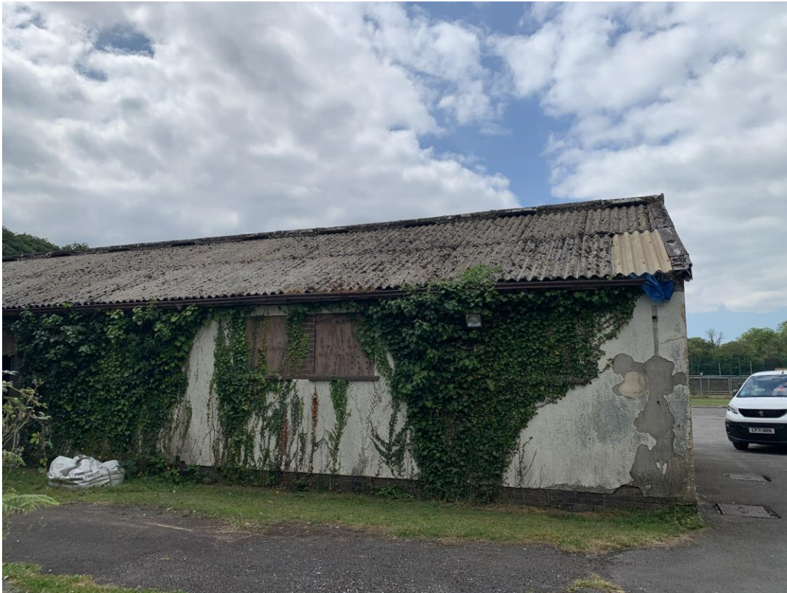
Photograph showing part view of the rear left corner roof. Previous patch repairs undertaken with a GRP sheet covering. Moss growth and scaling of the roof covering noted.
