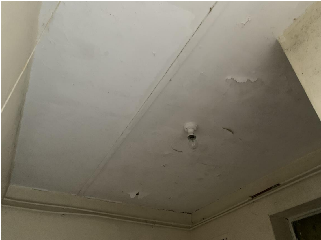
Photograph showing view of a fibre cement ceiling subject to extensive debonding of decorative finishes.
