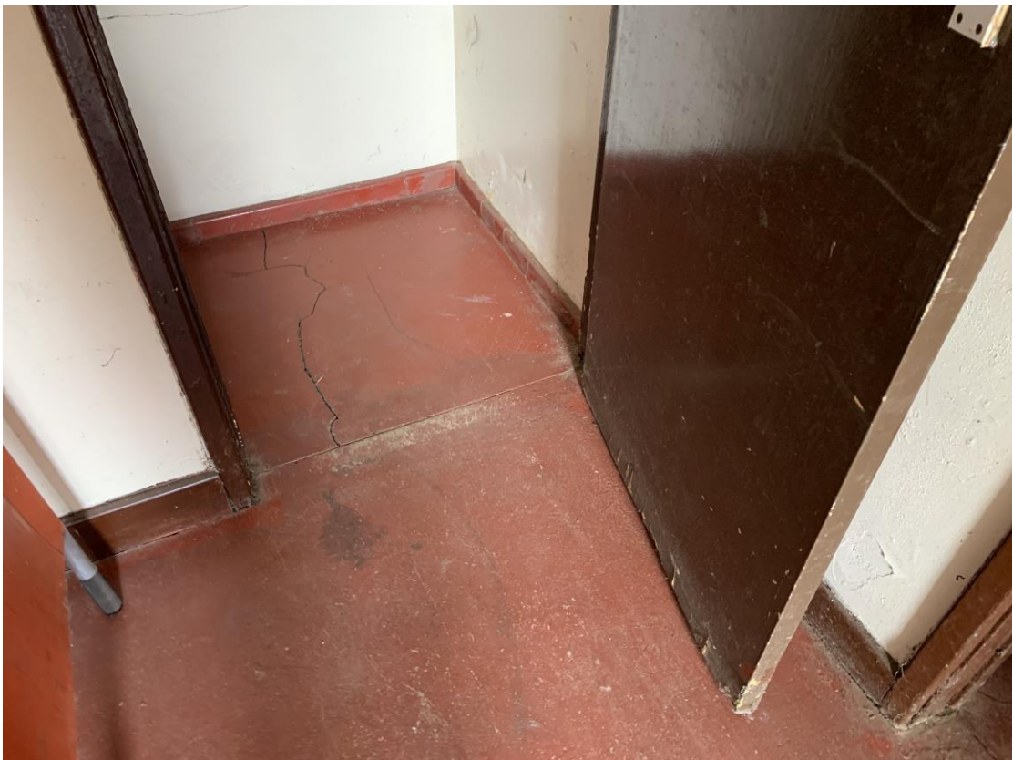
Photograph showing typical example of a crack within flooring.
