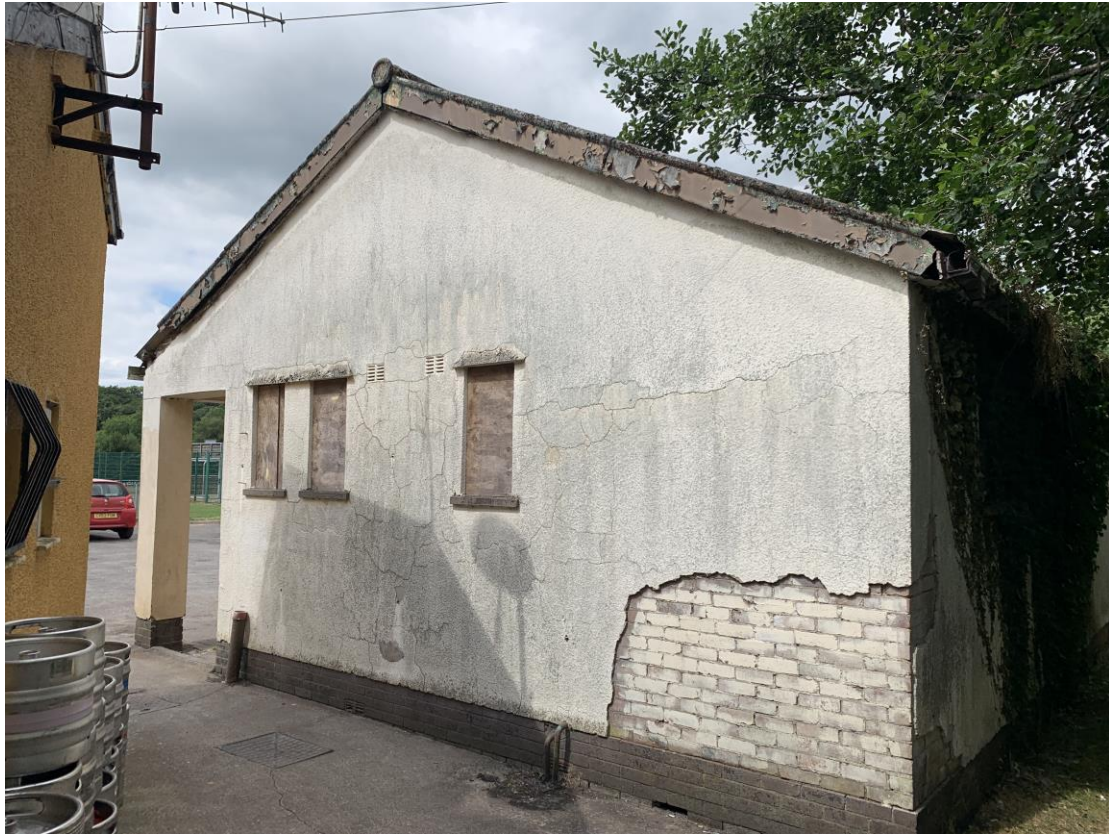
Photograph showing view of the right side gable elevation. Extensive cracking, hollow and de-bonded sections of render noted.
