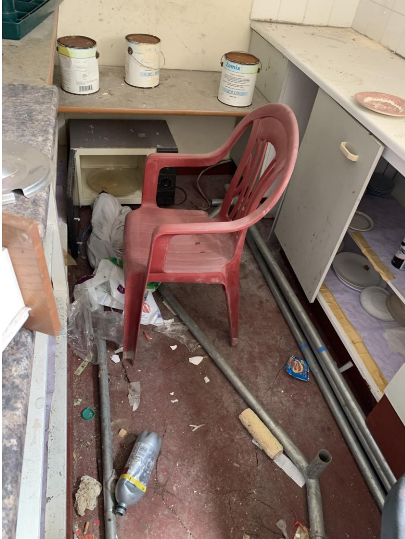
Photograph showing example of the poor condition and order to the fitted kitchen units.
