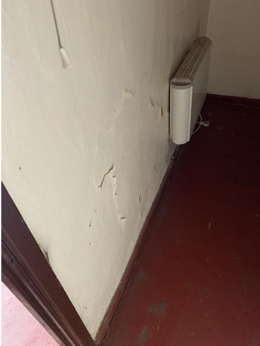
Photograph showing example of uneven surface finishes and de-bonded paint coatings along with low level contamination of plaster to internal walls.
