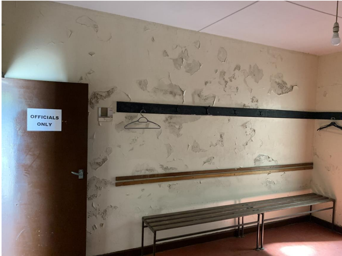
Photograph showing example of extensive contamination and de-bonded decorations to walls to changing room to left side of property.
