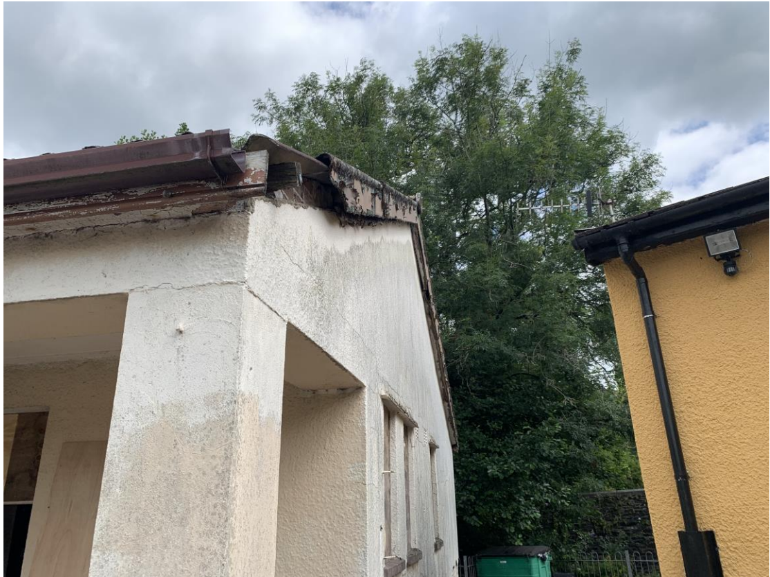
Photograph showing view of the front right corner gable where the fibre cement trim to eaves has been removed/missing.
