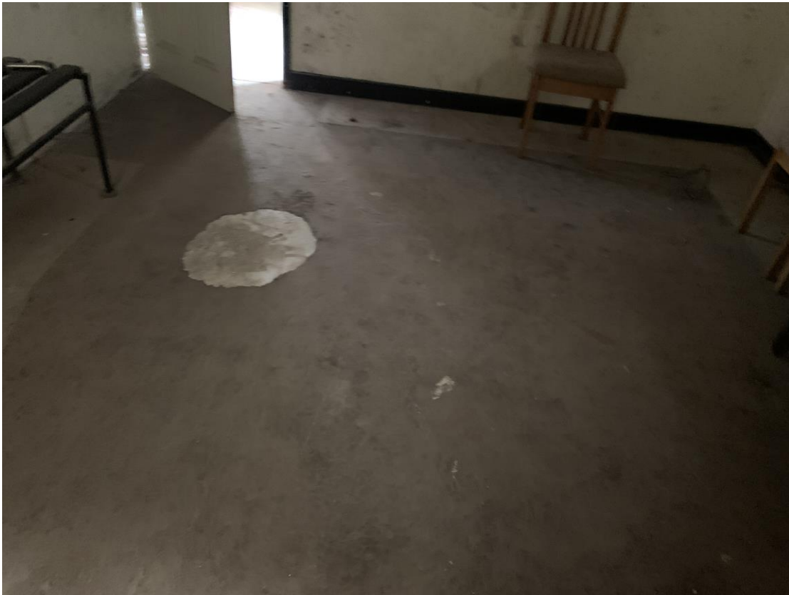
Photograph showing example of a proprietary floor coating that is subject to deterioration and de-bonding.
