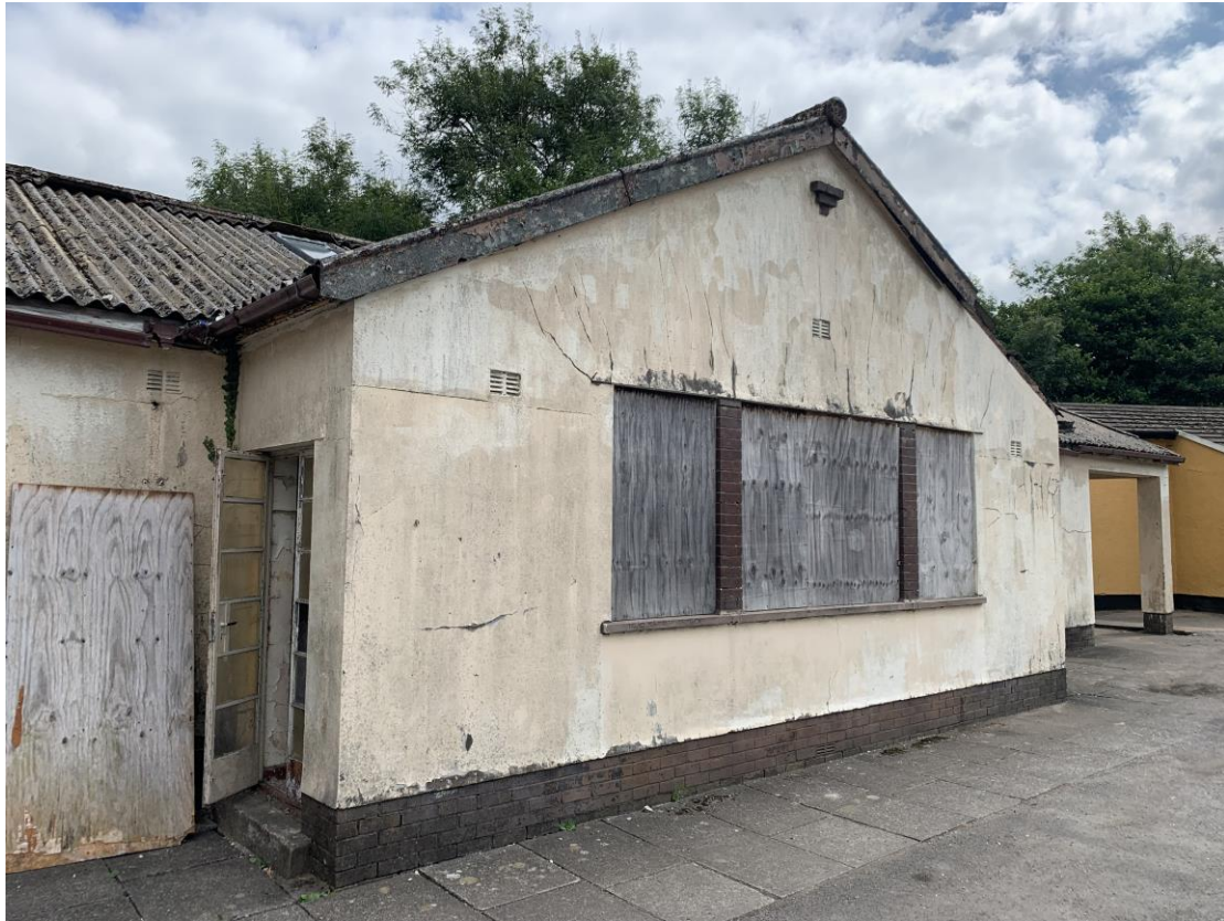
Photograph showing part view of front elevation where extensive cracking/de-bonding of the render was noted above windows.
