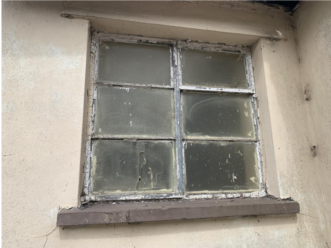
Photograph showing typical example of the window condition.
