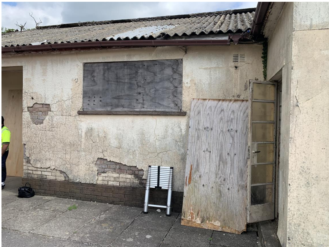
Photograph showing part view of the front elevation to left side. Cracking noted around structural members forming openings and also extensive cracking, de-bonding of the render finishes.
