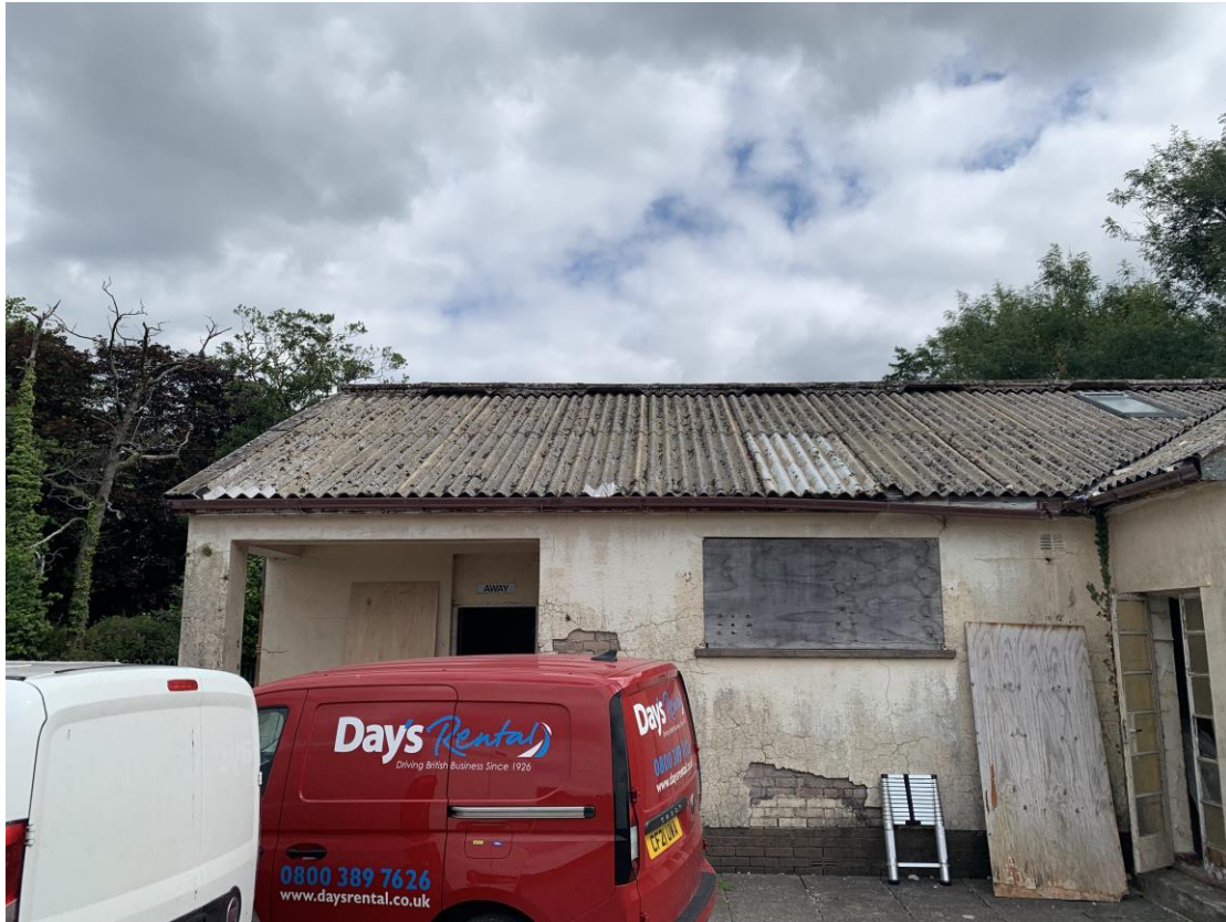
Photograph showing part view of the left hand side front roof slope. Impact damage along with previous patch repairs noted.
