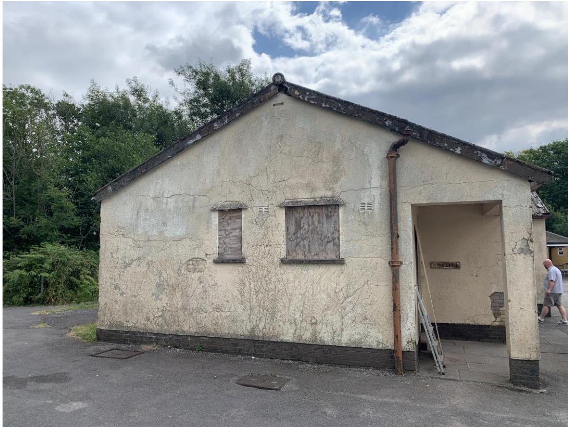
Photograph showing view of the left side gable elevation. Extensive cracking and de-bonding of render noted in several locations.
