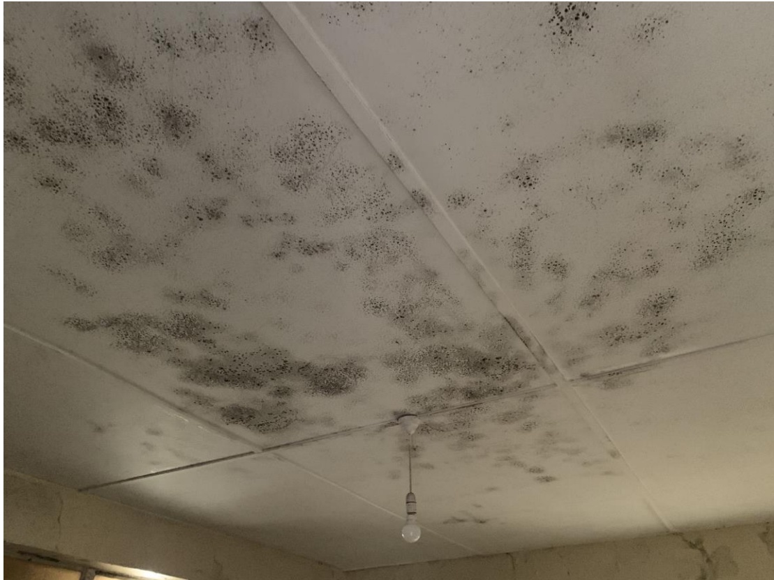
Photograph showing extensive staining, black mould growth and discolouration to ceiling to changing room to right side of property.
