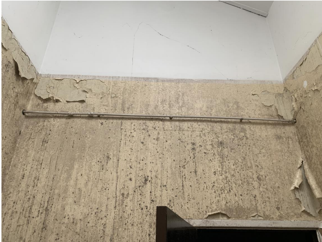
Photograph showing extensive de-bonding of decorative coatings along with black mould growth to wall finishes.
